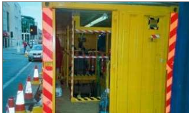
Figure 9 - HV cable jointing container
